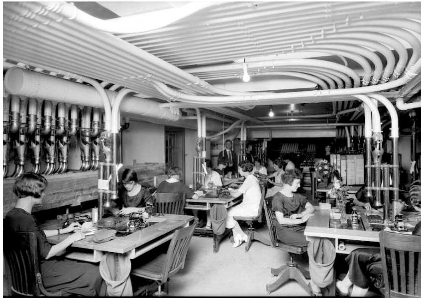
Pneumatic tubes, a critical component of the interoffice mail system.
